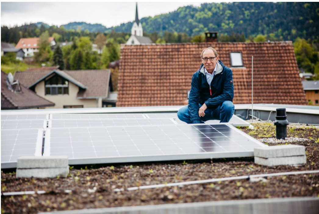
Figure 1 - Citizen solar power plant in Kennelbach (AT)
